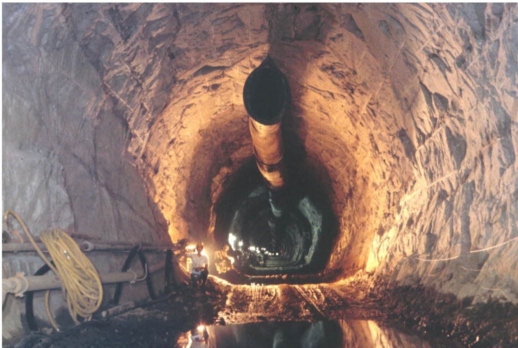
Figure 2 : Results achieved using well designed and carefully controlled blasting in a 7.2 metre tunnel in gneiss in the Victoria project in Sri Lanka. Photograph reproduced with permission from British Overseas Development Administration and from Balfour Beatty-Nuttall.
