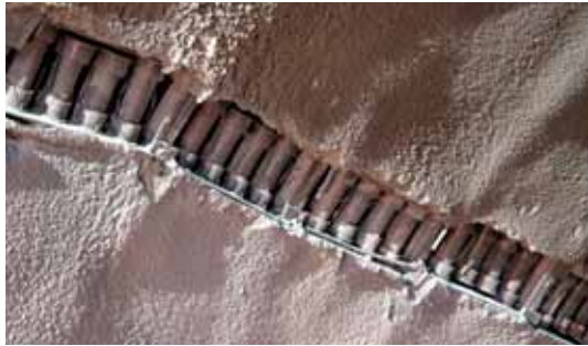
Above: a line of stress controller installed in one of the cross passages between the first and second tubes of the Metsovo tunnel
