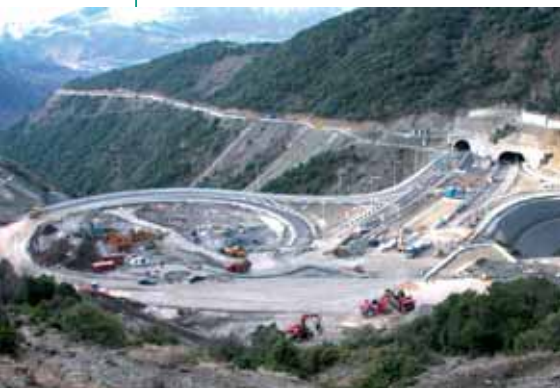
Above: an interchange and tunnel portals near the town of Metsovo in the Pindos mountains.
