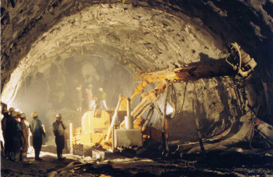
Figure 21: Installation of 12 m long 75 mm diameter pipe forepoles in an 11 m span tunnel top heading in a fault zone.
