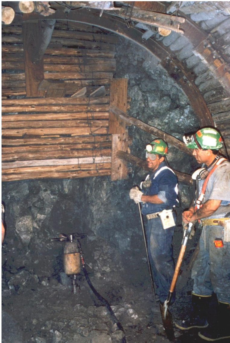
Figure 15: Installation of sliding joint top hat section steel sets immediately behind the face of a tunnel being advanced through very poor quality rock.
